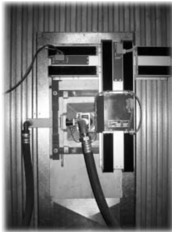
Second Generation Water Cannon installed at Southern Company’s Miller Plant on an 800 MW B&W front/rear wall-fired unit burning Power River Basin coal.
