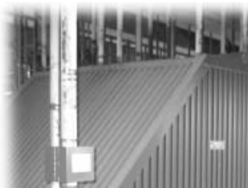
SmartGauges installed on hanger rods at TVA's Cumberland Plant as part of an EPRI project.
