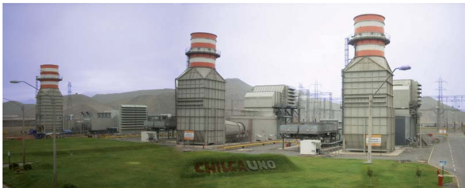
Existing gas turbine exhaust stacks at the Chilca Uno power plant, Peru
