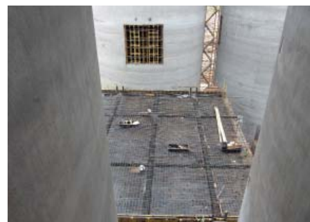
Conditioner building within the fly ash silos
