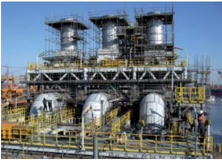
Three WHRU installed on Modec's Guara FPSO
